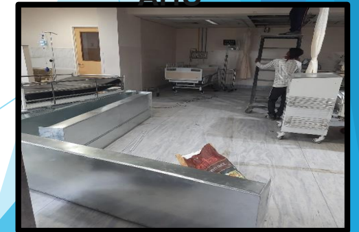
Modification in ducts for Two OT's ran with one AHU
