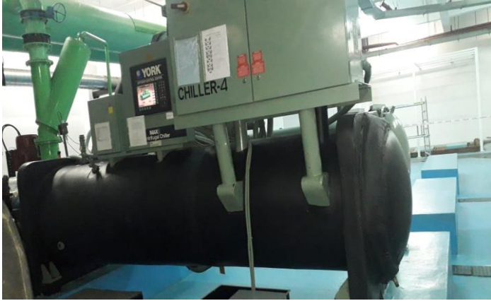
Chillers on VSD
