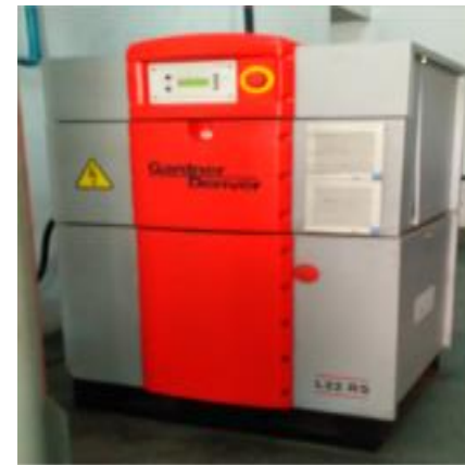
VFD operated Air Compressor
