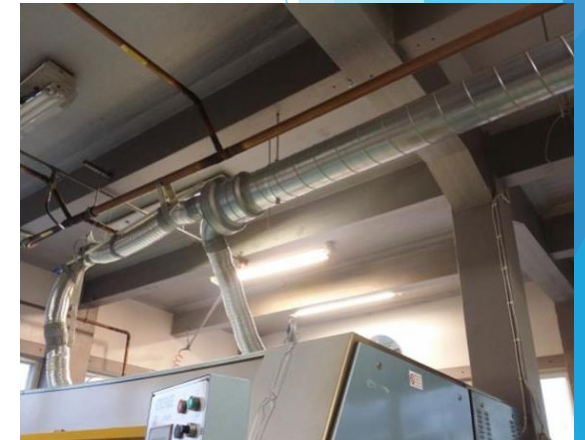
Thermal recycling in Laundry
