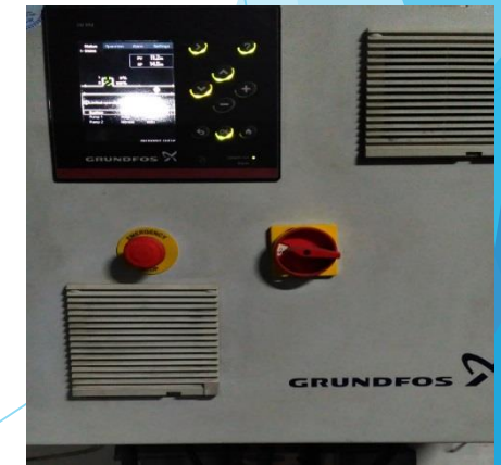
VFD on AHU's
