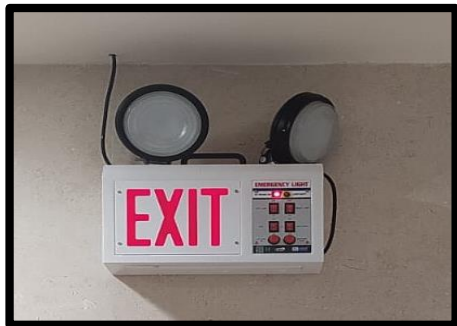
Battery Operated Emergency lights in Corridors/stairs
